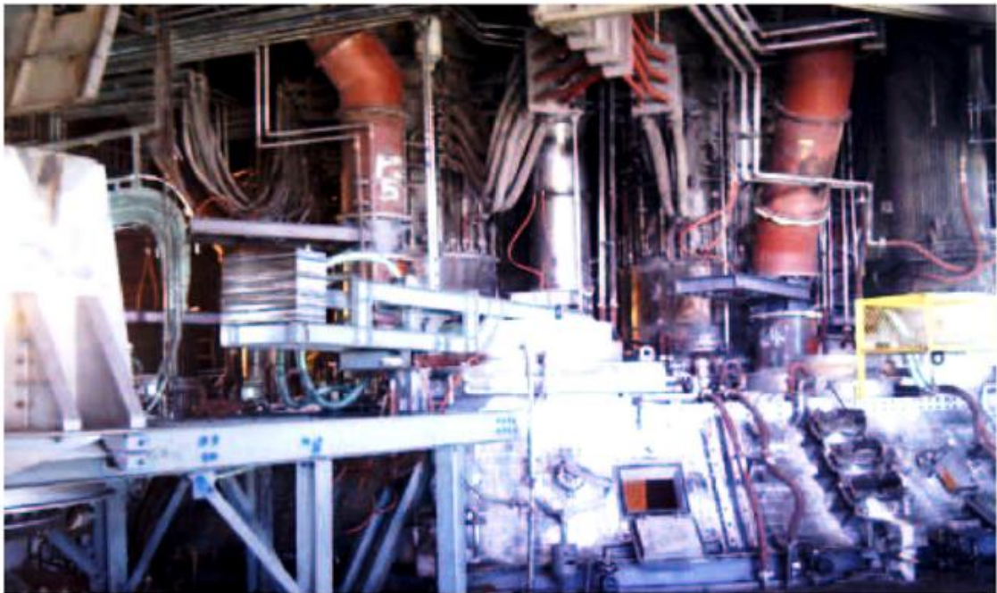
Metix's upgrade of IFM's two 66 MVA FeCr furnaces had already enabled the company to achieve 12% of its target production cost savings by January of this year.
